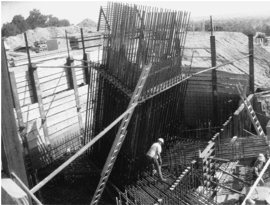
Construction is ongoing at the site of the Air Force Memorial in Washington, D.C.
